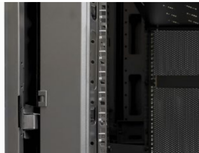
Vertical Cable Management Rails Opened
