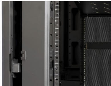
Vertical Cable Management Rails Opened
